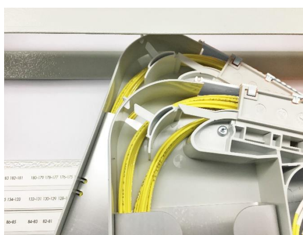
10.4.6 Close internal cable/pigtail clips and inner bend control in the shelf.
